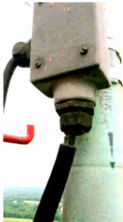
Fig. 1: During the re-lamp job, your climber can inspect your tower for problems like this where an AC cable for a radome heater is coming loose.
