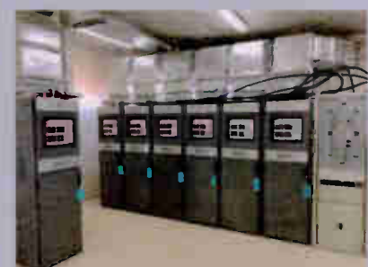
Nautel NV Series FM transmitters, part of an earlier TRT infrastructure modernization project, are shown in Dikmen, Ankara, Turkey.
