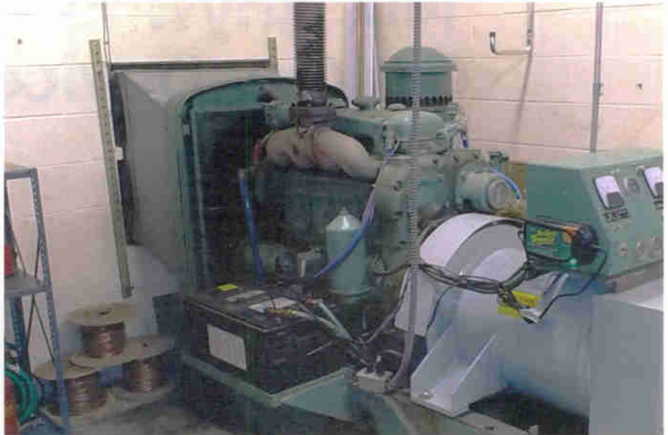
Fig. 1: This genset recently kept WNIS running for 38 hours.
