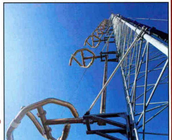
Photo courtesy of Kilowatt, Inc.
