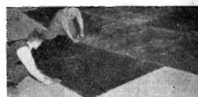
Laying a Celotex roller floor. Ordinary mechanics can apply the big, strong 4 by 12-foot Celotex Tempered Hard Boards direct to existing wood floors or sub-floors.
