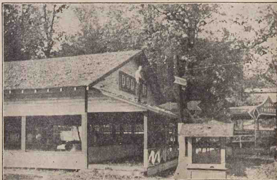
VIEW IN ROLLING GREEN PARK, between Sunbury and Selinsgrove, Pa., where a severe hailstorm dealt much damage on the afternoon of July 11. The Dodgem building shown was one of seven structures that required reroofing after the storm, said Manager R. M. Spangler. The man is pointing to hailstones as big as golf balls that smashed thru the roof. Even autos with turret tops were damaged.
