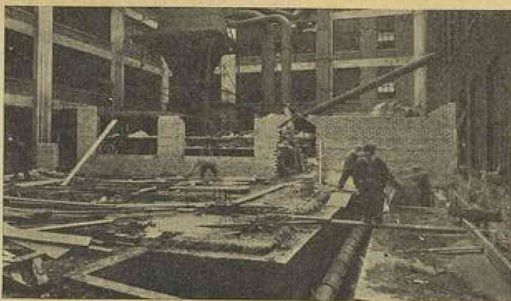
WITH SHOW-TIME RAPIDLY APPROACHING, officials of the Rock-Ola Manufacturing Corporation report they are preparing the biggest surprise they have ever had. Workmen in the above picture are busy constructing a new addition to the factory. It is said that special huge presses will be installed to facilitate the new heavy production schedule. "What is it? You'll see it at the 1941 Coin Machine Show," say Rock-Ola officials.
