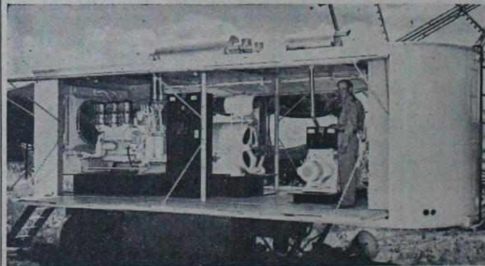
JACK RUBACK'S Alamo Exposition Shows have shifted to a Diesel light plant. Shown above is the new 180-kw. plant and Chief Electrician Jimmy Lukens. Plant was purchased from Stewart & Stevenson, of Houston, represented by Tobe McFarlan, and was delivered June 17 at Waco, Tex.
