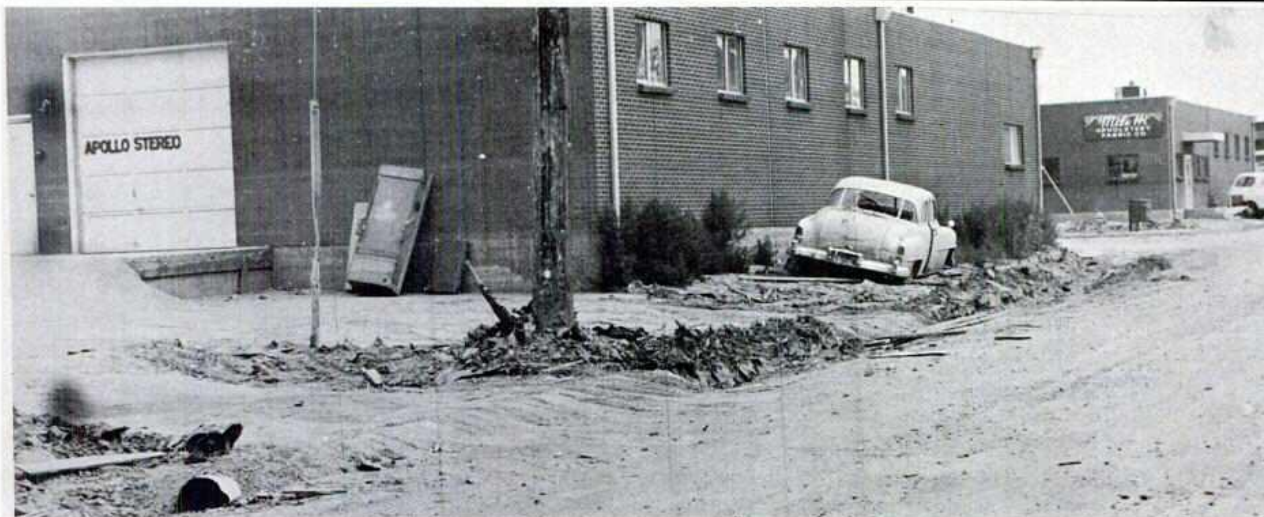
FLOOD CURRENTS hurled this automobile against the south side of the Apollo-Stereo Building, causing extensive damage to the structure. The Apollo-Stereo firm also sustained heavy damage to equipment stored in the building.
