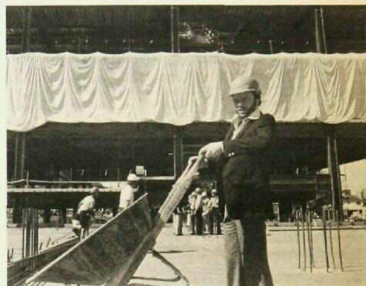
PITCHING IN—MCA Records president Bob Siner lends a helping hand at the site where the new MCA Records building is being constructed in Universal City, Calif.
