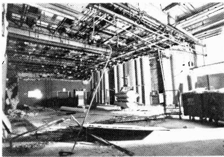
A Masterful Achievement. The control room area is just visible in the background of this photo of Mastersound Astoria Studios. The facilities, currently under construction, will be ready for business sometime in February.
