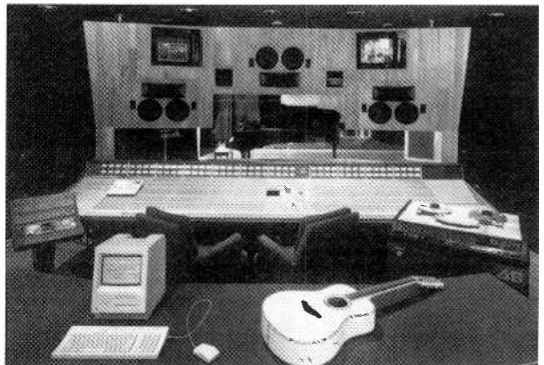
More Logic. Record Plant Los Angeles, a facility that is no stranger to Solid State Logic mixing consoles, has installed yet another of the high-end boards, this time in Studio 2. The desk shown here is an SL 4072 G Series , equipped with 64 channels, the G Series computer, and Total Recall automation.
