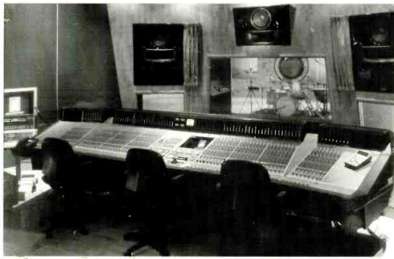
The Tracking Room at Masterfonics in Nashville, featuring Solid State Logic's top-of-the-line 9000J series console.
