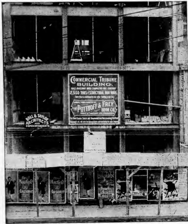
"CONSISTENCY, WHERE ART THOU?" The Cincinnati Commercial Tribune Building under process of erection. This paper opposes Billboards.
