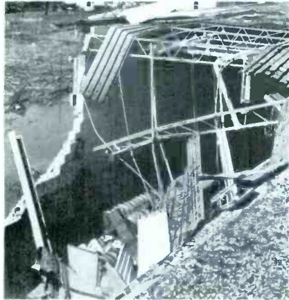
This view of the west wall also shows the collapsed roof area under which the electronics department was located. Repairs are currently underway in this section of the plant.
