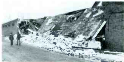
Here is a photo of the 200 ft. west wall which collapsed completely resulting in heavy exterior and interior damage, as well as personal injuries.
