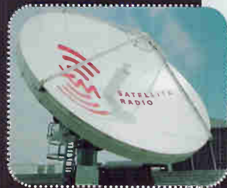
No Static At All: One of XM's two 23-foot uplink satellite dishes on the roof of the company's broadcast center.
