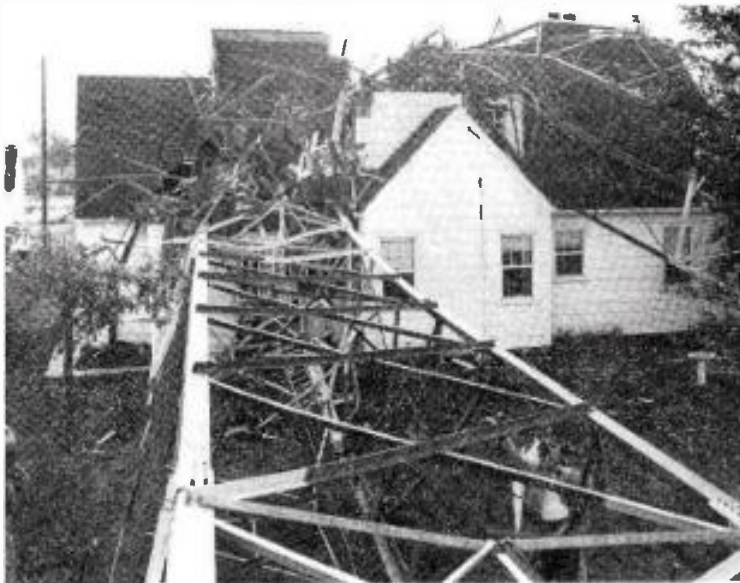
WHEN A TORNADO wrecked two towers of KMBC, Kansas City, Aug. 25, one of the towers, 544 feet high, fell on this house, 250 feet from the tower base. The antenna broke in the center before falling. Occupants of the house narrowly avoided injury [see story on page 42].
