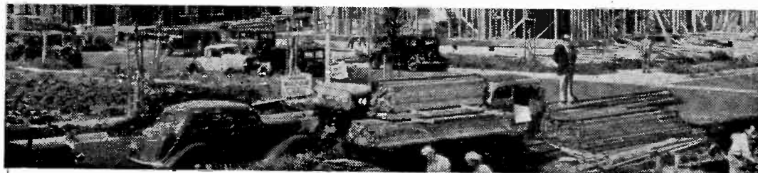
HOUSES ARE SPRINGING UP everywhere on West Coast. Typical of housing projects is this one in Los Angeles.
