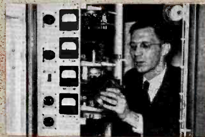
WALL-MOUNTED UNITS afford easy access to all tubes and wiring. Rear doors further increase ease of reaching all components. Illustration above shows portion of the aural transmitter's r-f driver unit.
