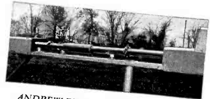
ANDREW FM-AM isolation section with cover removed, revealing two 3/8" FM transmission lines and expansion joints.
