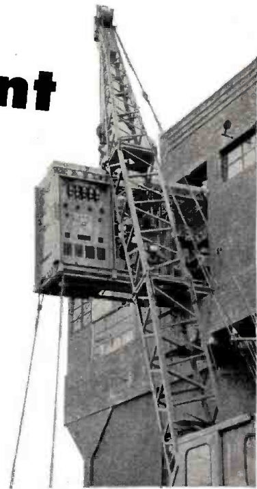
EASY DOES IT! This shot shows one of the units of the new KGW transmitter being derricked through a second story window of the transmitter house. The new installation will give KGW the most efficient transmitting equipment yet developed by the radio industry.
