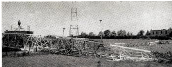
THIS wrecked transmission tower was the result of a sudden squall at Bloomingdale, Ill., last month that caused $50,000 worth of damage for WMAQ (NBC) Chicago [BROADCASTING, June 27]. This main transmission tower was erected only a month ago. The crash destroyed the transmitter antenna completely, but the station was back on the air in a minute and a half after Engineer Howard Lindsay switched on the emergency tower in the background.
