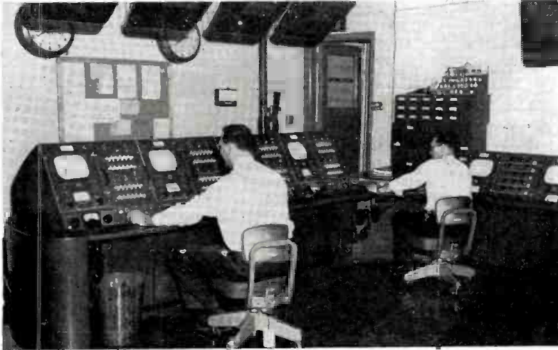
A portion of the new WOR-TV master control. Equipment at right is associated with film camera control.
