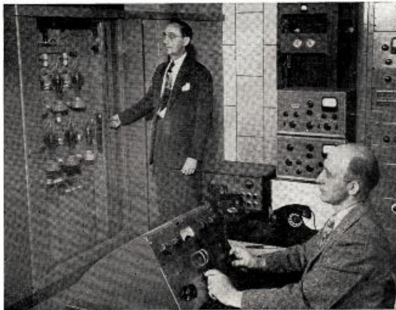
MANIPULATING the switch, Arthur F. Rekart (l), chief engineer, turns on the KXOK-FM St. Louis new 10 kw transmitter located in the Boatmen's Bank Bldg. in downtown St. Louis. Robert V. Nicholas, assistant, operates the control panel. New facilities, in operation since April 27, enable the station to broadcast with a radiated power of 70 kw in a 17,500 square mile area. Its new tower rises 574 ft. above street level. KXOK-FM, affiliated with Transit Radio Inc., broadcasts continuous music-news-weather programs to 1,000 buses and streetcars of the St. Louis Public Service Co.
