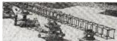
Shown above are portions of the apron, the steel frame and several of the dollies.
