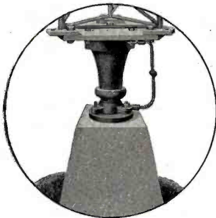
Base insulated central pier showing "Mast-Base" or "Pivot" type base insulator with Spark-Gap.
