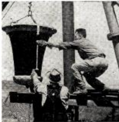
It's out with the old insulator and in with the new at the tower-raising of WHO Des Moines—an operation which required boosting some 200 tons skyward and four hours of actual work.
