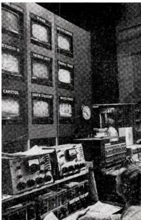
NBC-TV inaugural coverage was master-minded from control rooms in the Wardman Park Hotel, headquarters of the network's WRC WNBW (TV) Washington, D. C. outlets. Master control board shows monitored pickups from several vantage points where NBC maintained positions for its 15 cameras. William R. McAndrew, NBC-TV special events chief, directed coverage of Capitol ceremonies and parade festivities.
