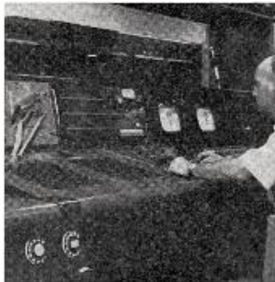
Nerve center • The tape reader at left feeds information into the data processing and storage section of automation equipment which in turn performs all switching operations.
