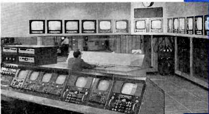
WJAC-TV's engineering facilities boast the newest electronic equipment to deliver the best television for its viewers---and buyers
