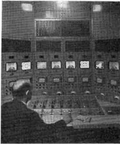
The closed-circuit control room, which transmits pre-recorded programs and commercials to CBS offices, can handle eight channels simultaneously.
