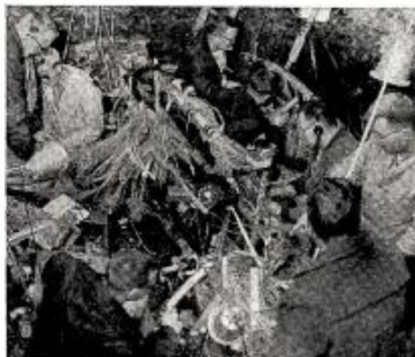
A line crew in the cable pit, painstakingly splicing thousands of wires in one cable to their mates in another.
