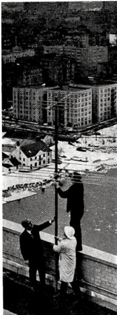
High above the Harlem River, workers for CATV Enterprises align an antenna at the head-end site atop a 28-story apartment building.
