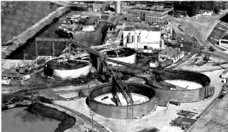
Water Treatment Plant at Republic's hot and cold strip mill complex recycles more than 100 million gallons of water daily. Original cost: $18 million Additional water clarifiers: $6 million
