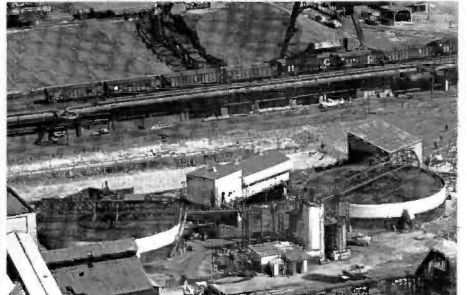
As part of Republic's water quality control program, additional facilities are being constructed at #5 and #6 blast furnaces to permit reuse of treated water.
