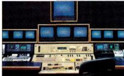
DIGITAL FINISHING ROOM
