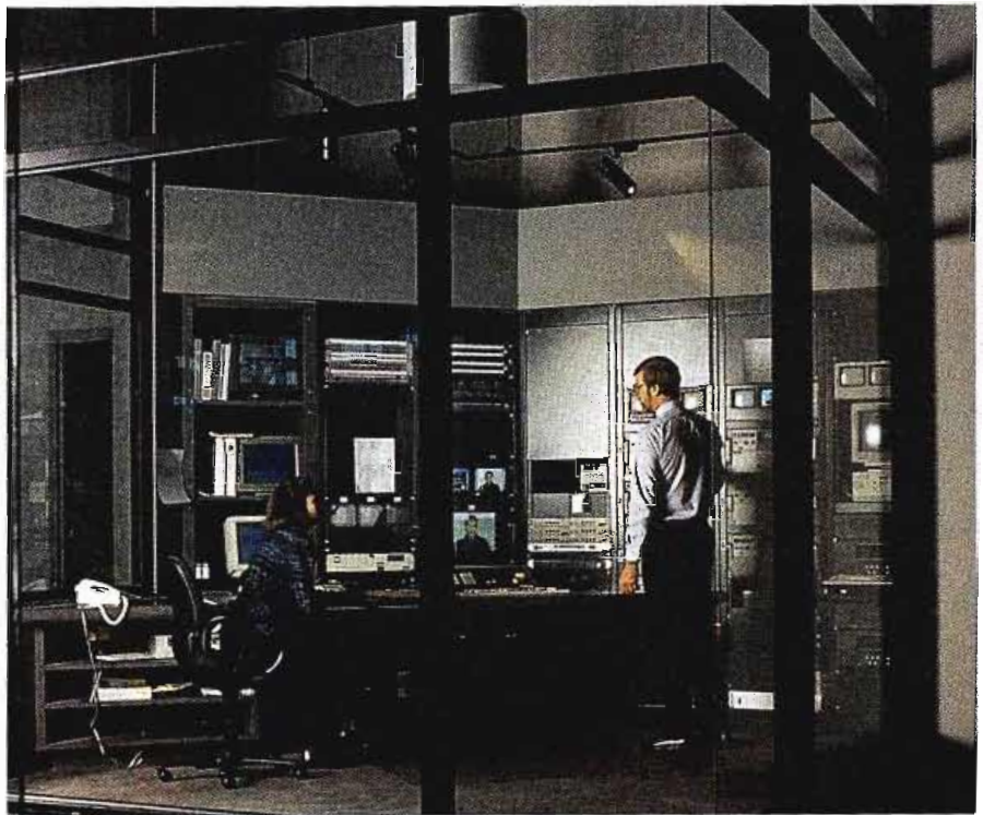
Master control for ME/U at the new uplink facility (Julie Trujillo and Larry Cole)
