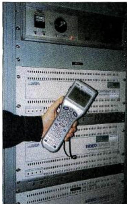
Warner Cable-Milwaukee's ARM (Automated audit Routing and resolution Method) combines this hand-held computer with a database tracking system to combat cable theft.
