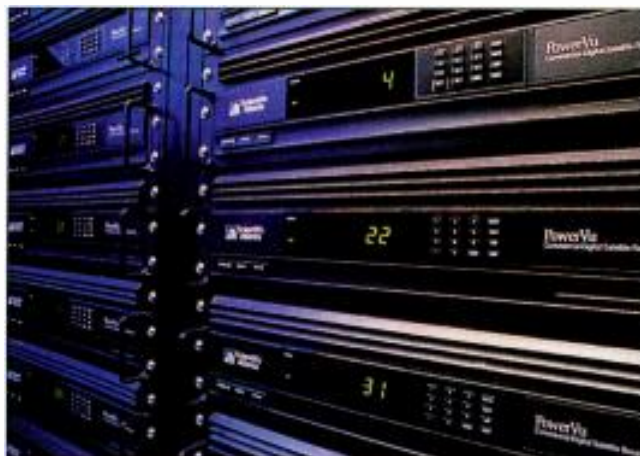
Discovery is equipping its Asia Broadcast Centre with S-A's PowerVu compression system.
