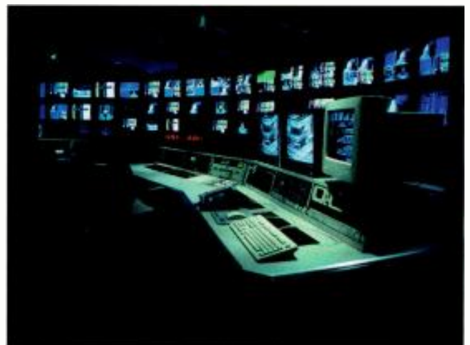
NBC's virtual broadcast at work – with AT&T's highly reliable, FASTAR®-protected digital multimedia solution (including data, voice and audio).
