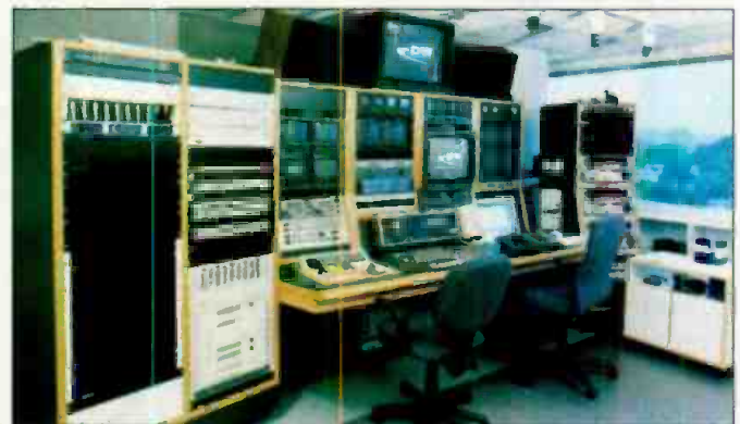
Communications Engineering Inc. designed and engineered Deutsche Welle's new technical facility in Washington.
