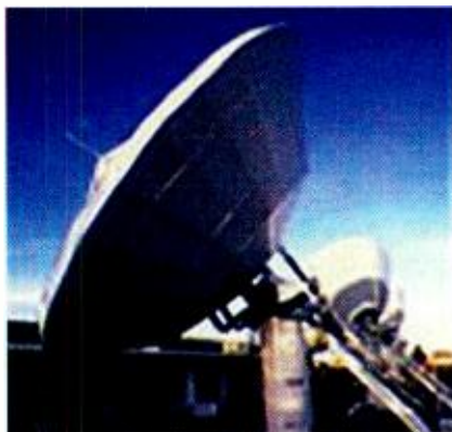
At the NDTC in suburban Denver, TCI’s control room and satellite facilities will be operational, even if the power fails on New Year’s Day. Officials plan to play it safe by having enough fuel on hand for emergency generators.
