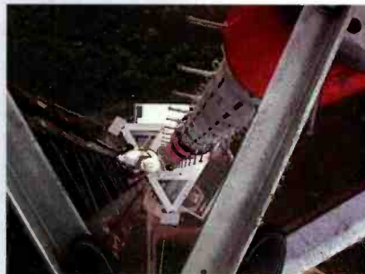
A Dielectric antenna (at left and below) broadcasts digital signals for KHOU-DT Houston, which spent nearly $6 million on the conversion.
