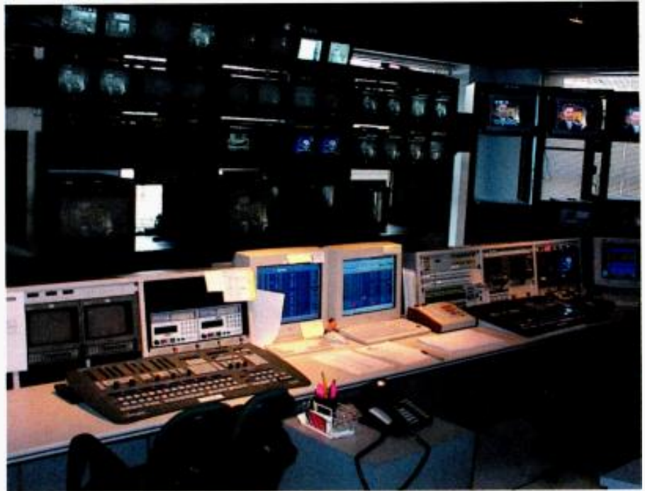
WLS-TV's master-control area features separate Saturn master-control panels for 720p HDTV (in foreground) and standard-definition channels (background).
