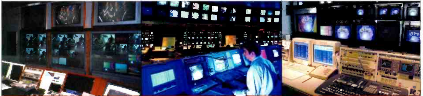
WETA-TV Washington's master control (left) makes use of Harris automation. A BSkyB supervisor (center) can monitor and access all channel outputs across the system, which has centralized alarm functions. Florical's automation system (right) keeps WLS-TV Chicago running.
