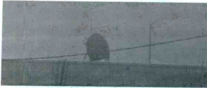
Small STL microwave dish on the roof, shown here along side regular UHF antennas, sends video and audio to transmitter site.
