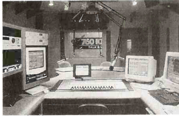
PR&E's Integrity™ digital console installed at KFMB-FM San Diego
