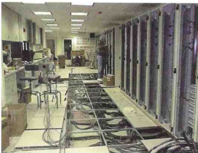
The master control room which will operate as the brain center for all five stations
