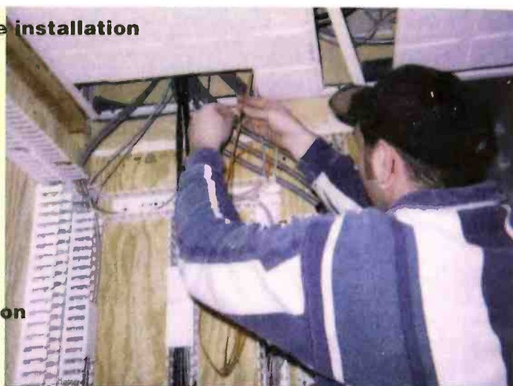
Mike Kane, Halik's Remote Coordinator, wires up the Ethernet and fiber optic lines in Buffalo for the Klotz Vadis platform.
