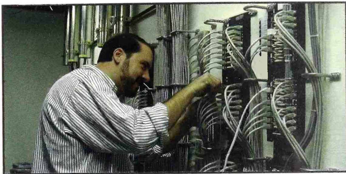
Jeff Depolo , a contract engineer, puts the finishing touches on studio interconnect wiring at the Radio Systems/Capstar Roanoke project.
