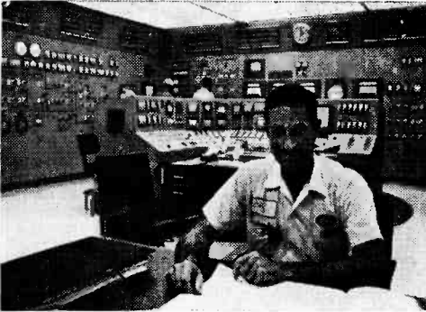
One of San Onofre's five watch engineers, Pat Riley is empowered with making go/no-go decisions in event of trouble. His job: to make sure that everything remains AOK.
