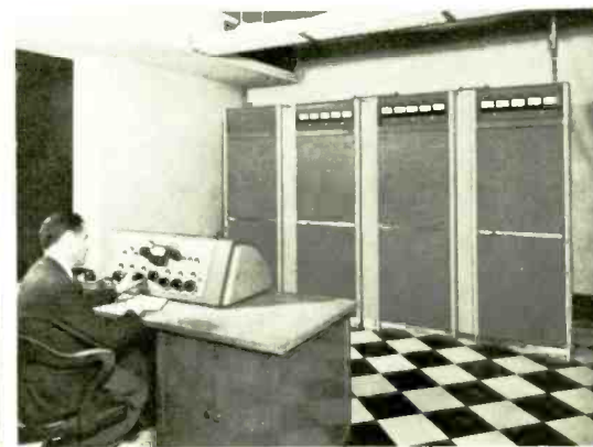
Top: Control Room, Russ Taylor
