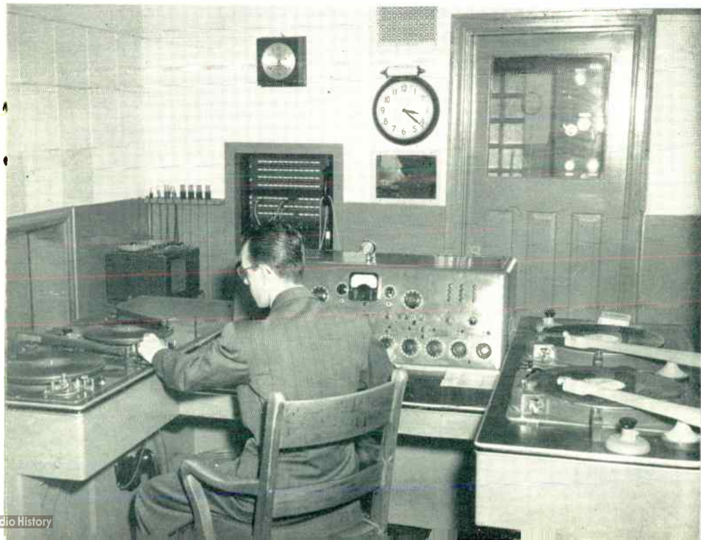
Operator Doug Fry at master control panel
